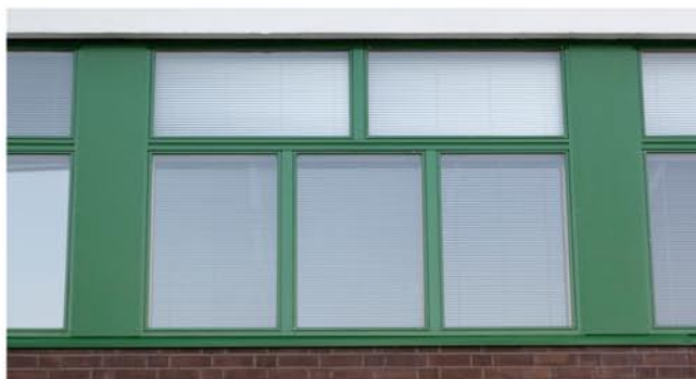
The Rastaala school, with its white enamelled windows in four shades of external colouring; infill panel windows. Each window features five parts in one frame.
